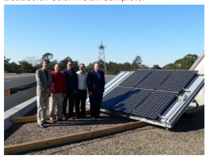
Lafayette Utilities System BeauSoleil's Solar Installation
